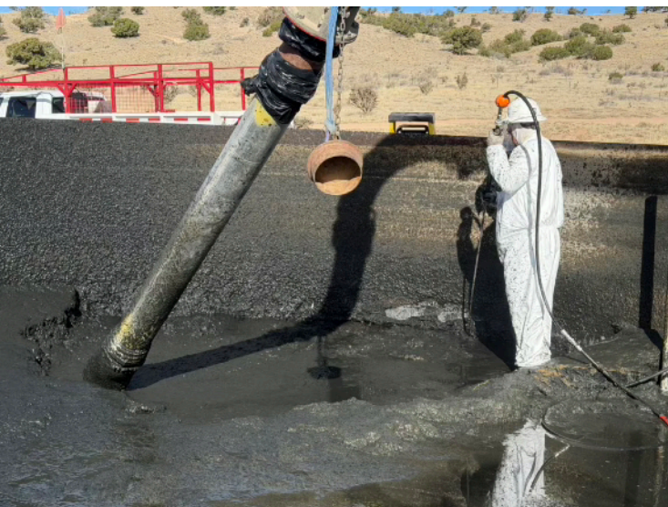
The depth (and quality) of the deposit in the tank can be seen in this picture.
