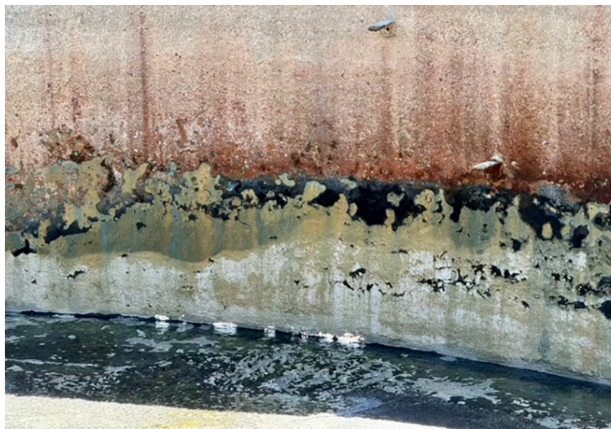
Once the tank sides had been pressure cleaned, corrosion and pitting of the tank wall became more obvious.
