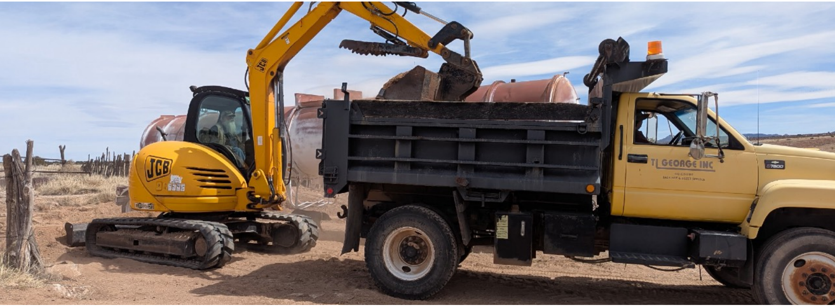
Before the trailer tank could be set, the site had to be cleared. HOA President John Mruskovic loads the HOA dump truck with his excavator.
